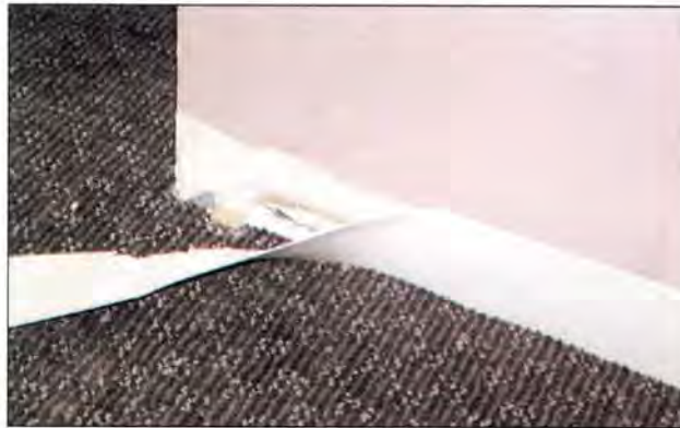
Removed base shows a common wall defect which is disguised by TightLock's thick wedge profile.
